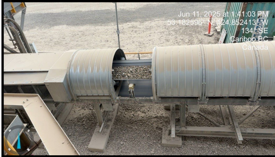
Photo 19: Plant Site Conveyor moving Ore through Crusher Circuit
