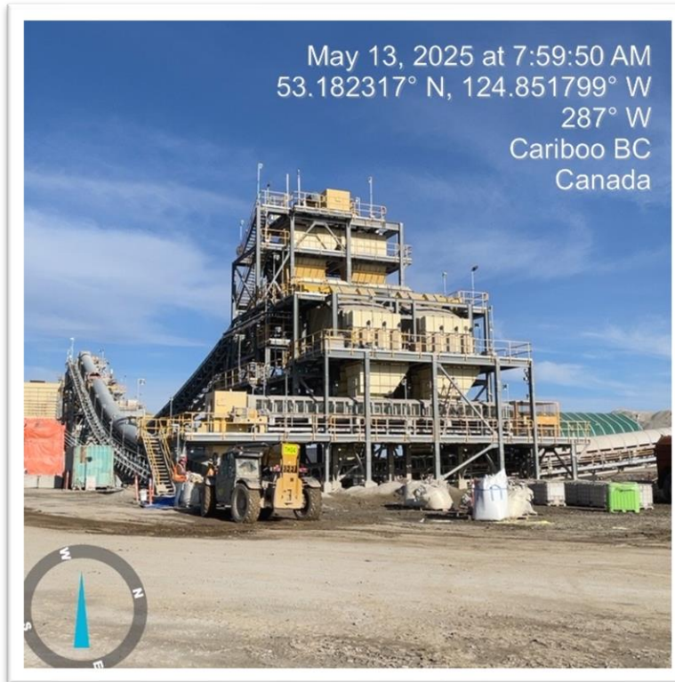
Photo 26: Plant Site IPAC Dust Suppressant and Water Spray Bar
