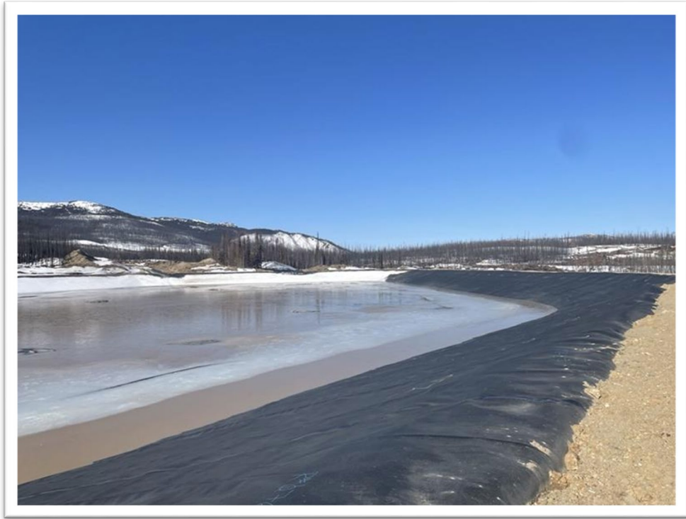
Photo 14: Low Grade Ore Pond Textured Lining
