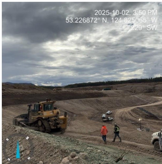
Photo 18, 19 & 20: Fresh Water Reservoir
