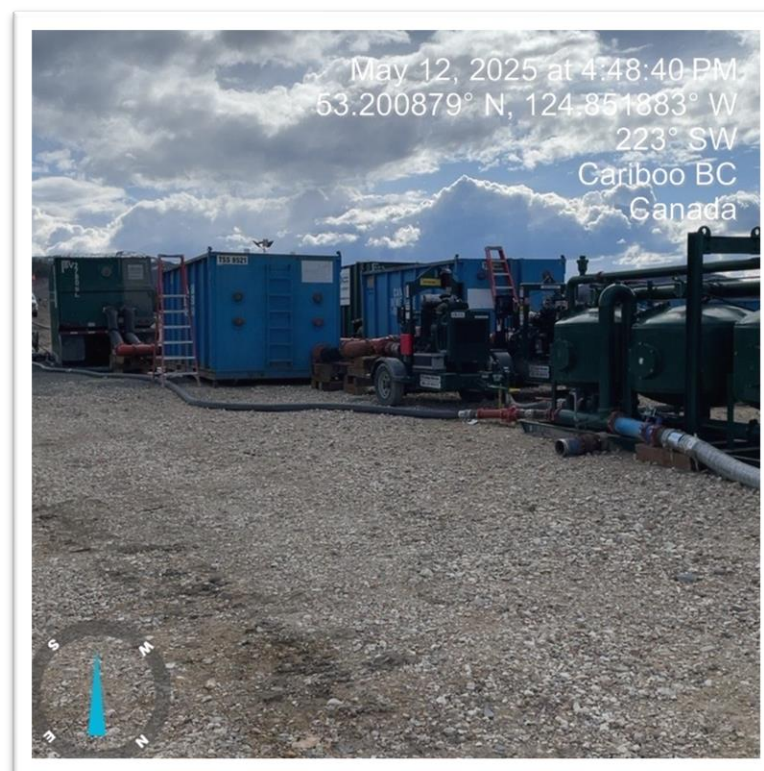
Photo 22 & 23: Water Management Pond Clarifiers
