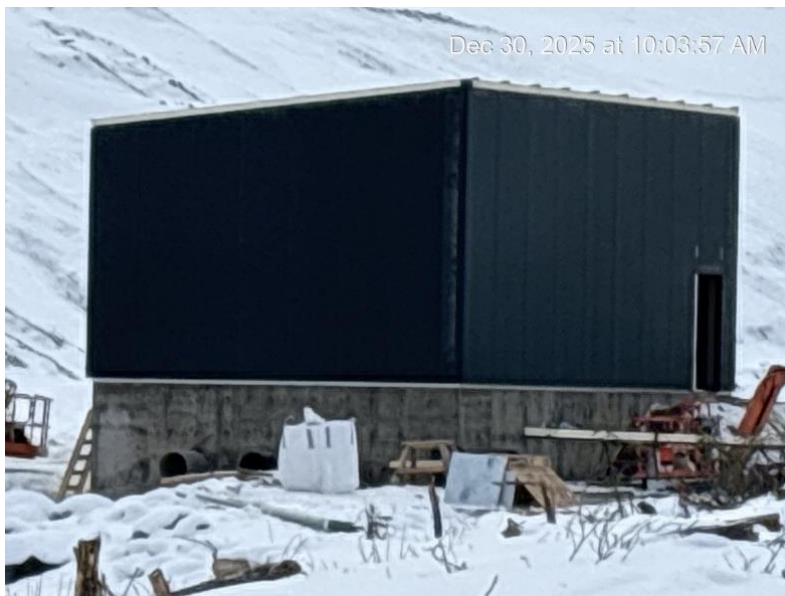
Photo 36: Pump House at FWR
