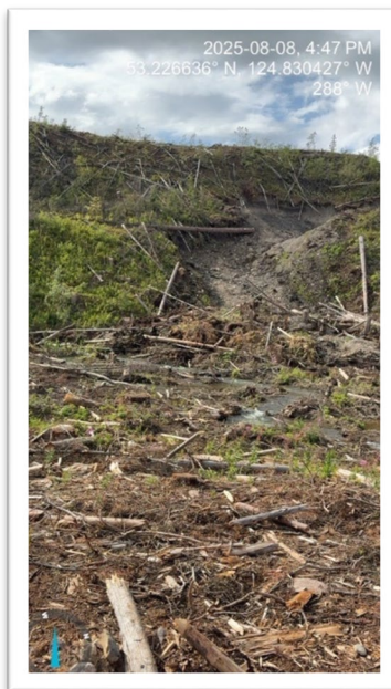
Photos 21 & 22: Fresh Water Reservoir Landslide
