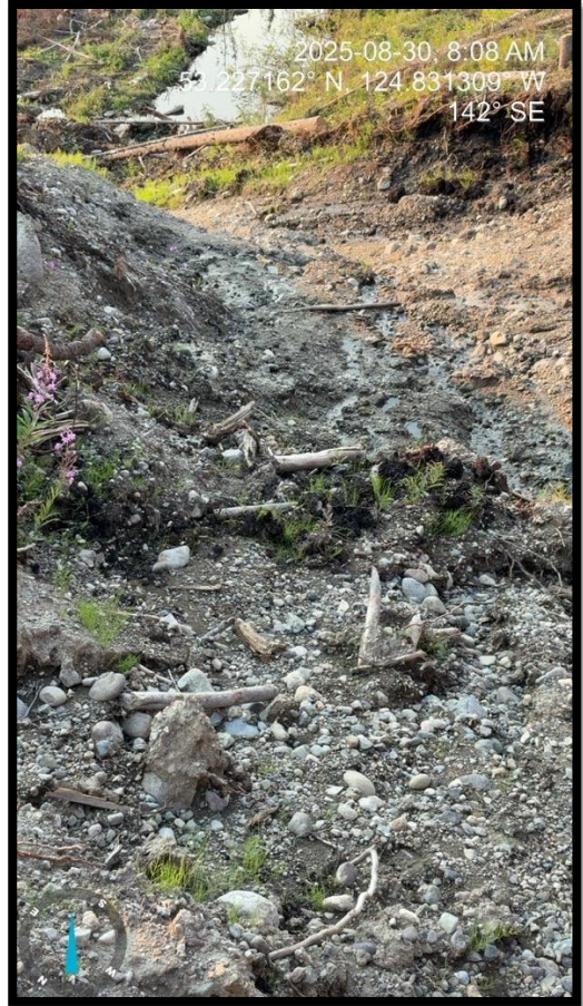
Photo 11: Spring runoff at the slide
