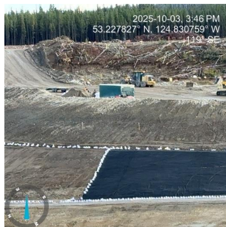
Photo 29, 30, & 31: Fresh Water Reservoir
