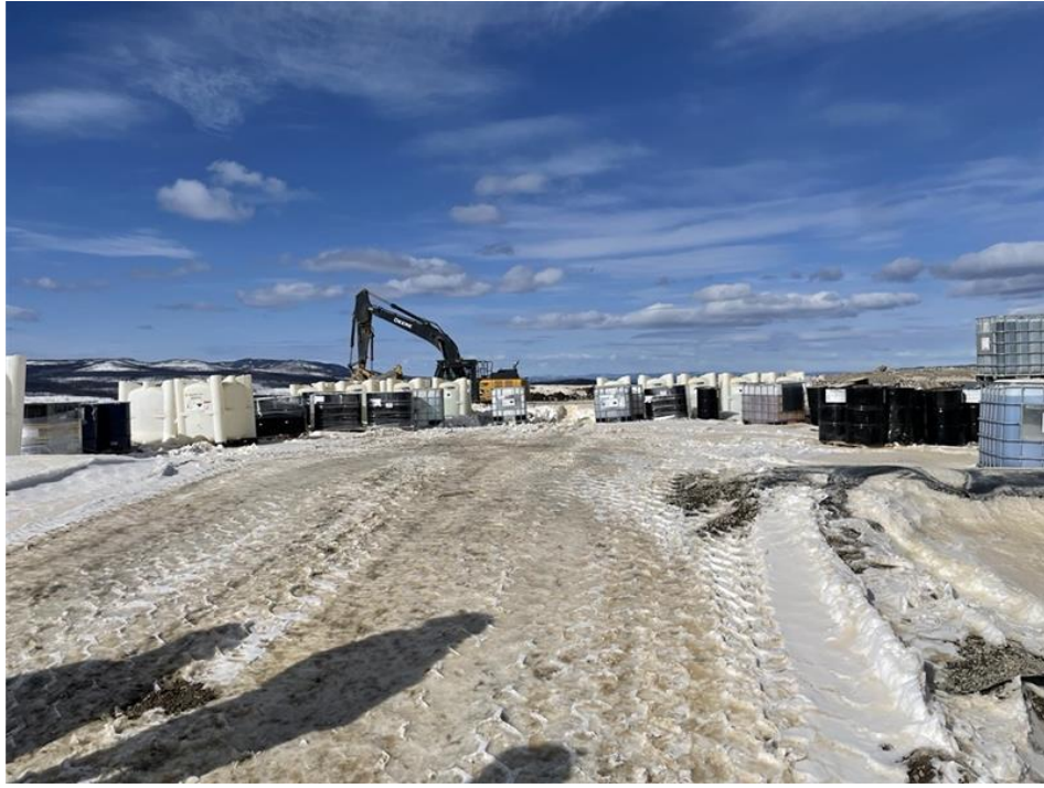
Photo 8: Lined Containment Berm for Chemical Storage at Plant Site
