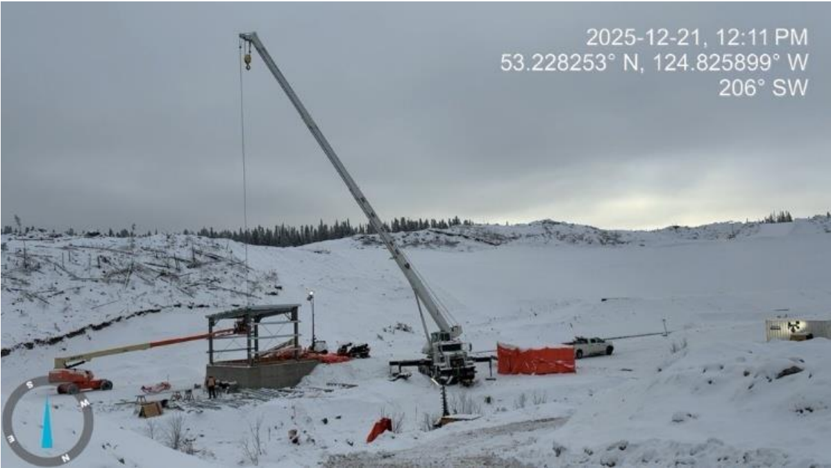
Photos 14 & 15: Pump House Station at Fresh Water Reservoir
