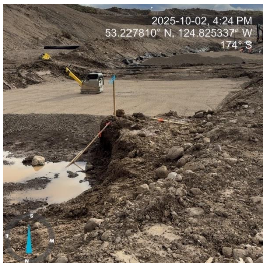
Photo 21, 22, & 23: Fresh Water Reservoir
