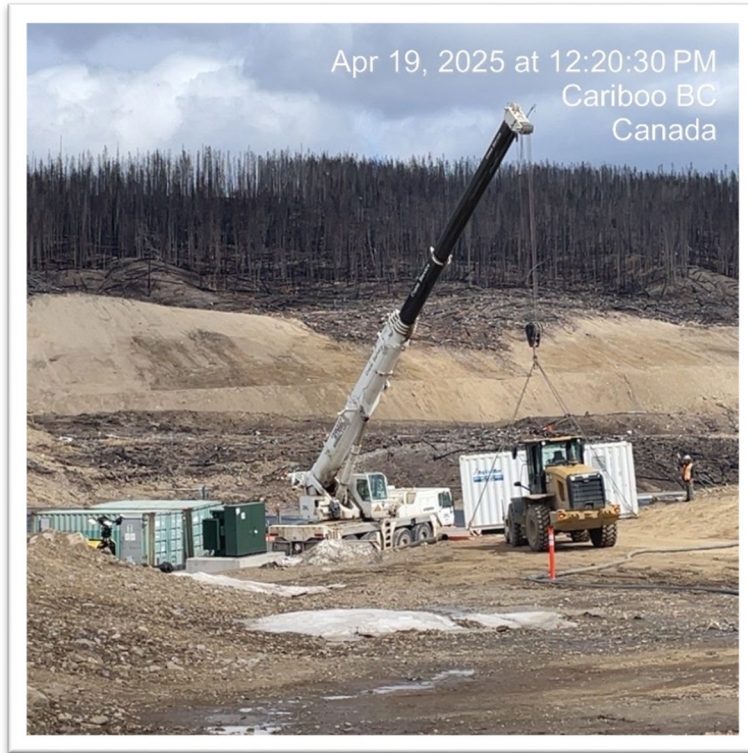
Photo 30: Pump Sea Cans Being Staged at Central Water Transfer Pond
