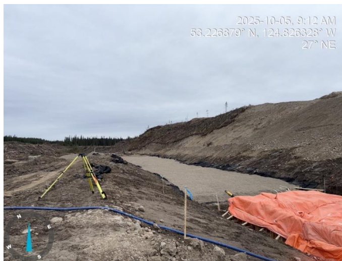
Photo 45, 46, & 47: Fresh Water Reservoir
