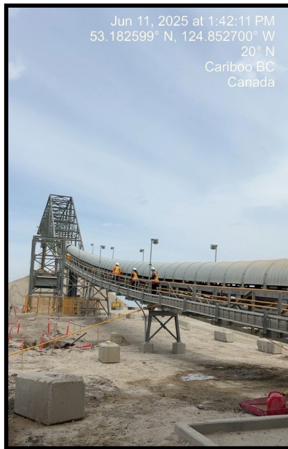
Photo 20: Plant Site Conveyor
