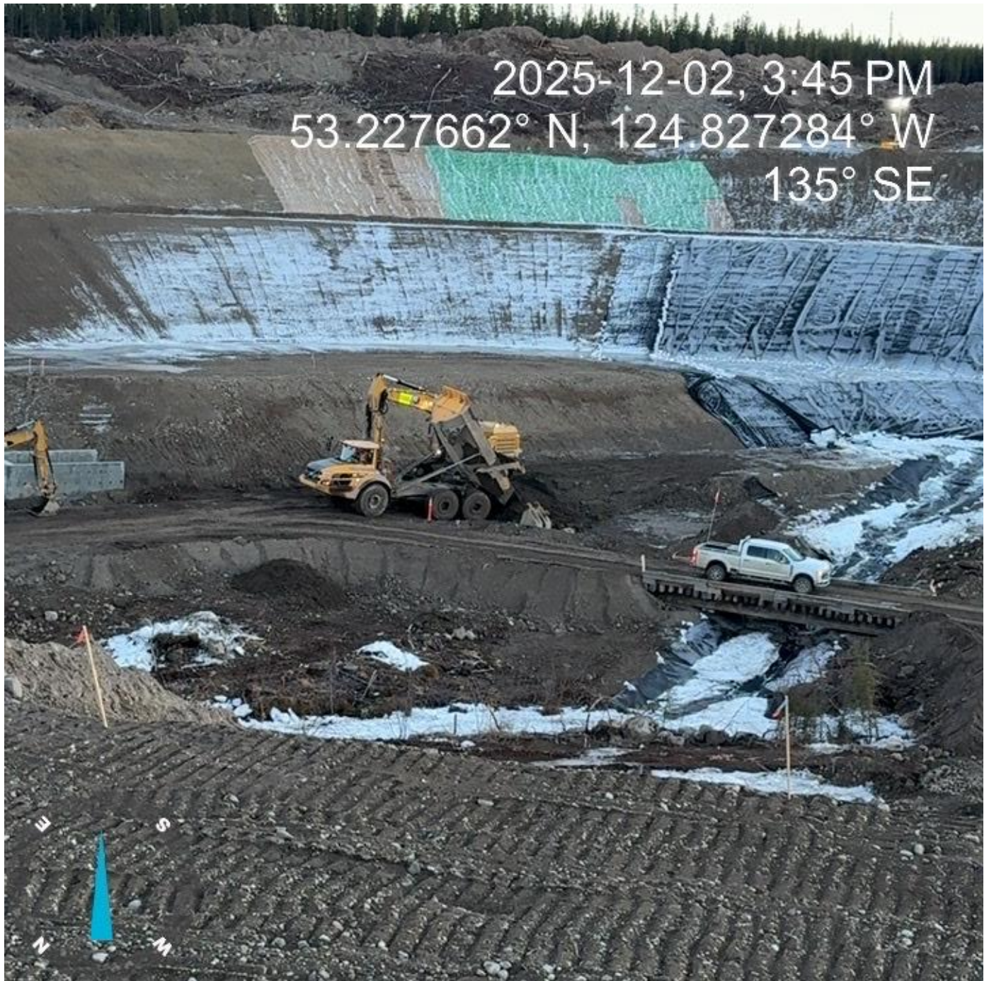
Photo 4: Fresh Water Reservoir
