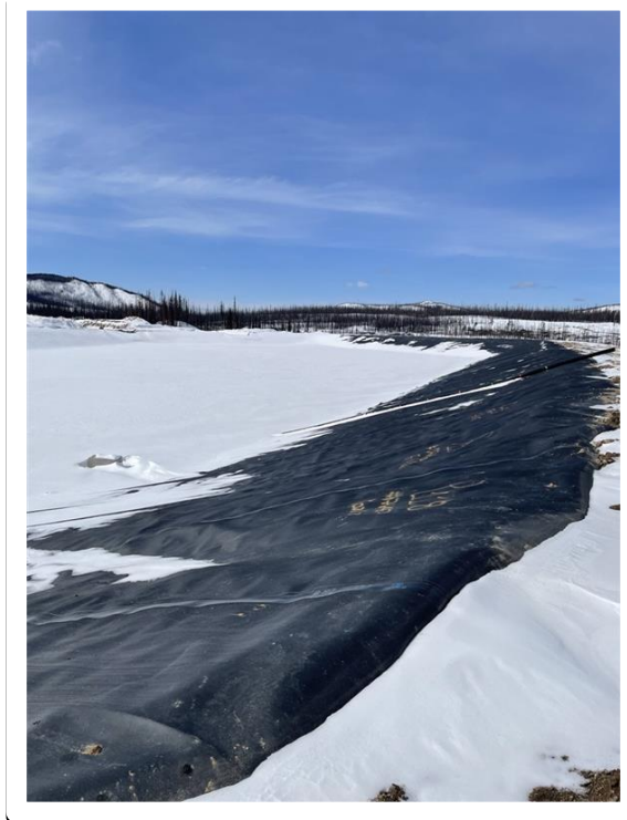
Photo 5: Low Grade Ore Pond Textured Lining
