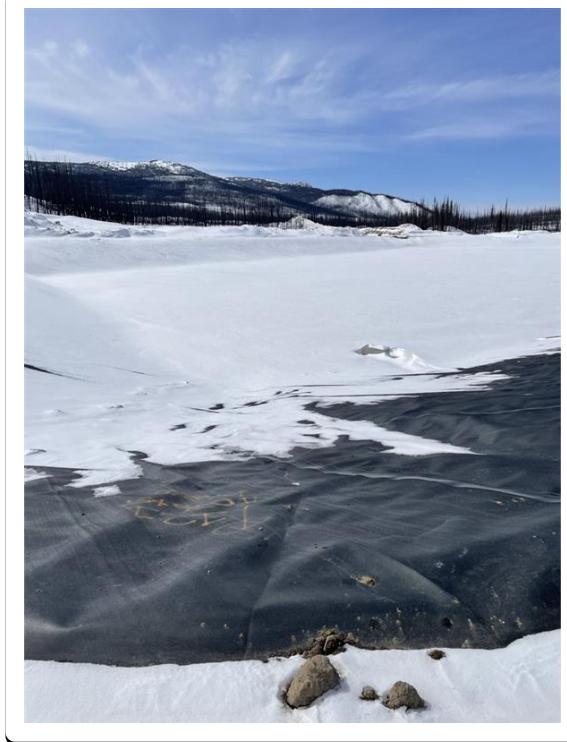
Photo 6: Low Grade Ore Pond Textured Lining
