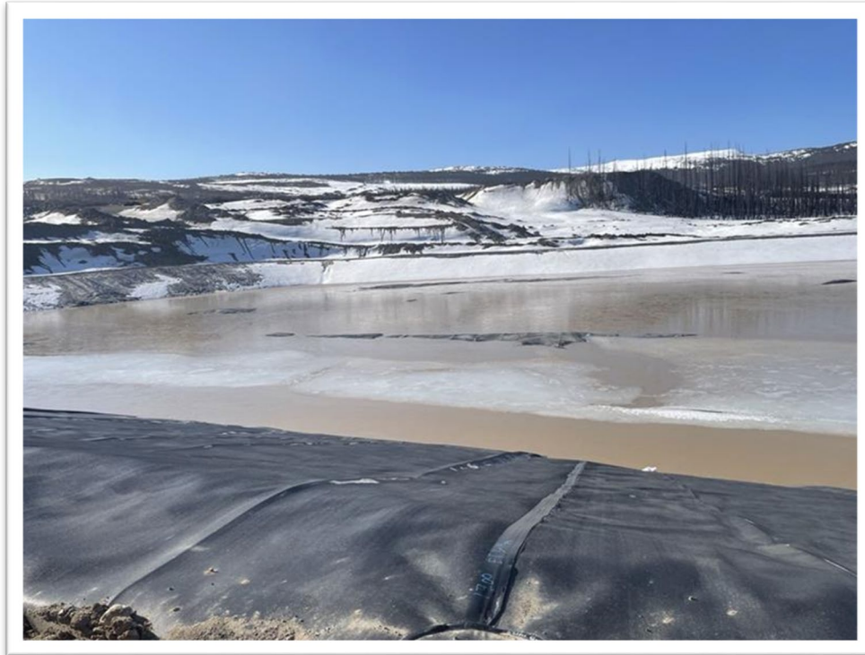
Photo 13: Low Grade Ore Pond Textured Lining
