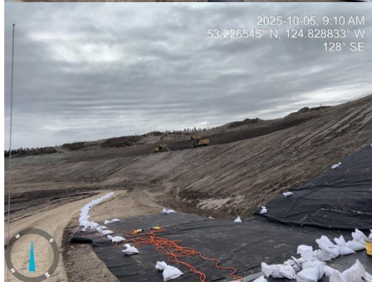
Photo 42, 43, & 44: Fresh Water Reservoir
