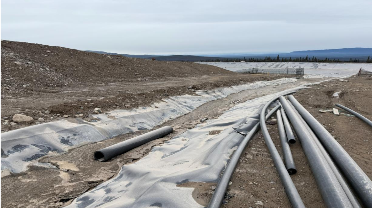
PHOTO 15 – SCC debris and sediment accumulation, looking north (Photo taken on November 12, 2025)
