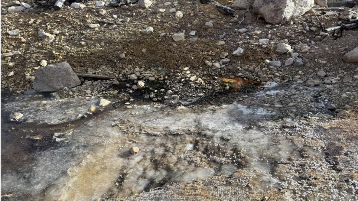
PHOTO 9 – Seepage observed at the downstream toe of Lake 16 Diversion Berm (Photo taken on October 13, 2025)
