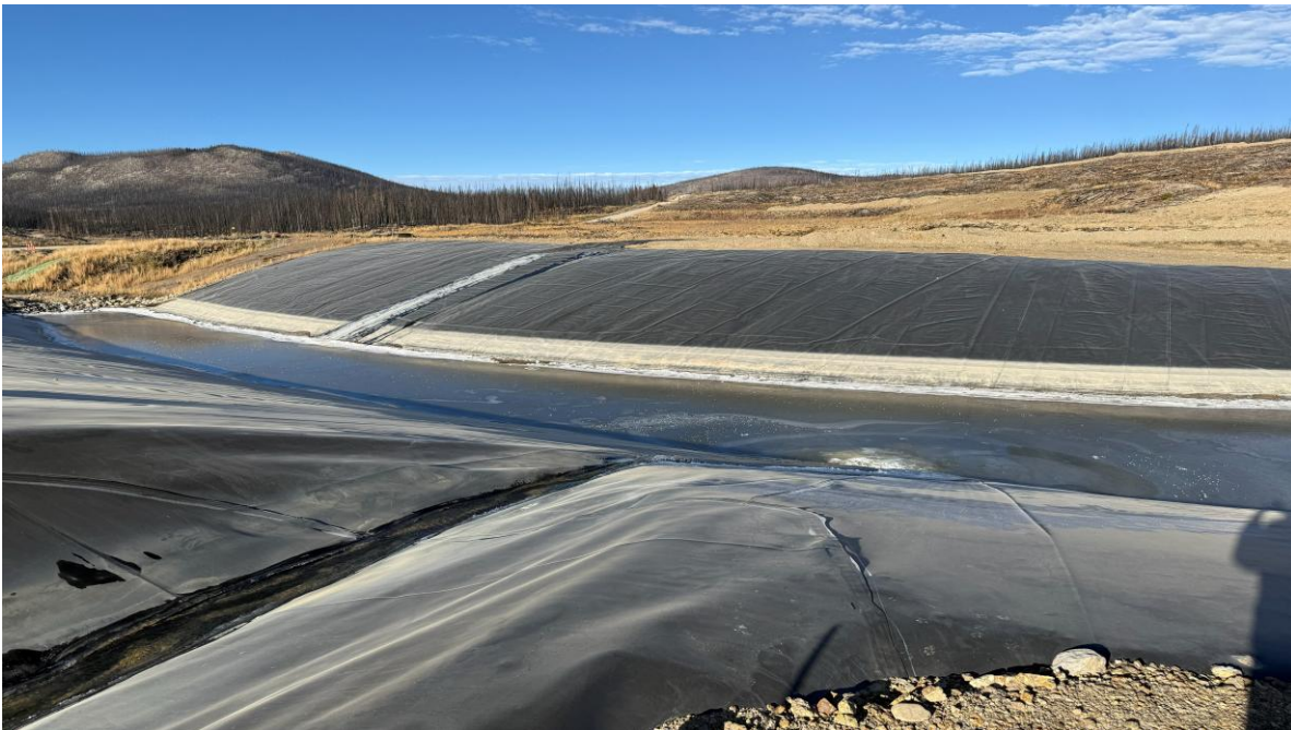
PHOTO 14 – SCC discharge into CWTP, looking southwest (Photo taken on October 13, 2025)
