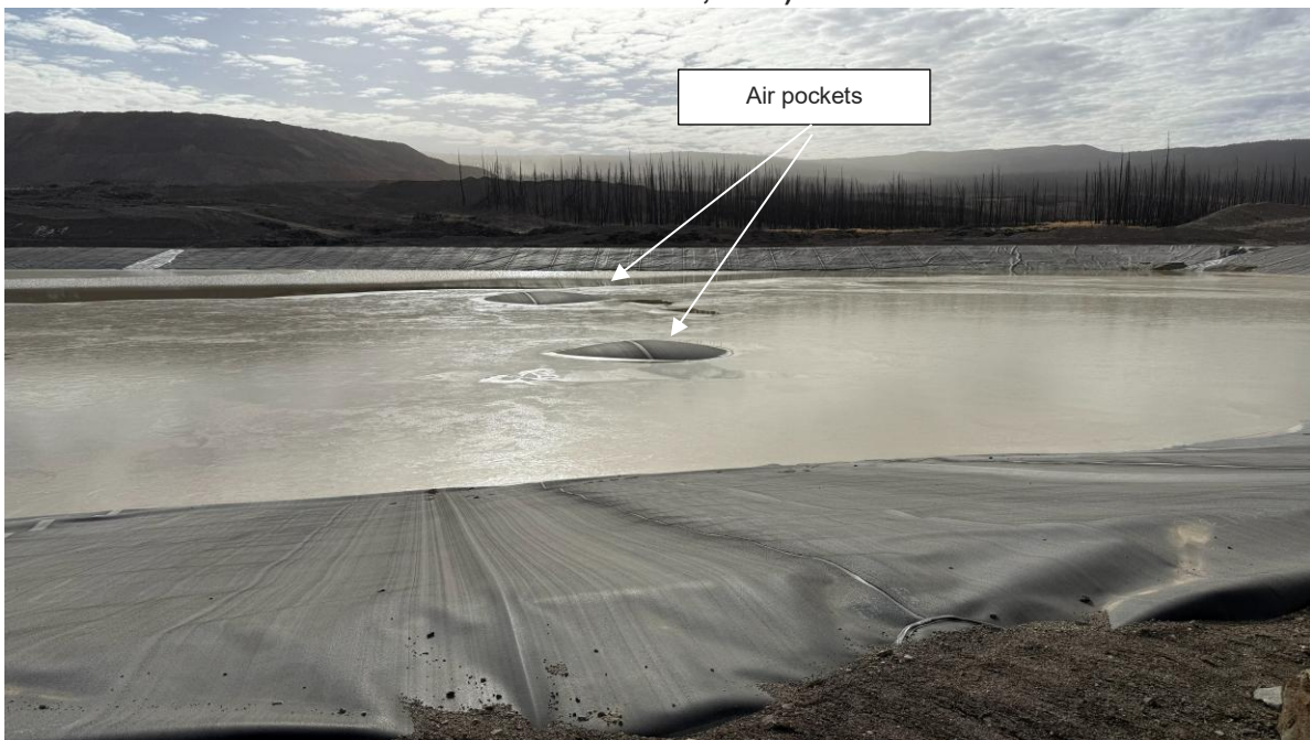
PHOTO 12 – LGO CP HDPE liner air pockets, looking south (Photo taken on October 13, 2025)
