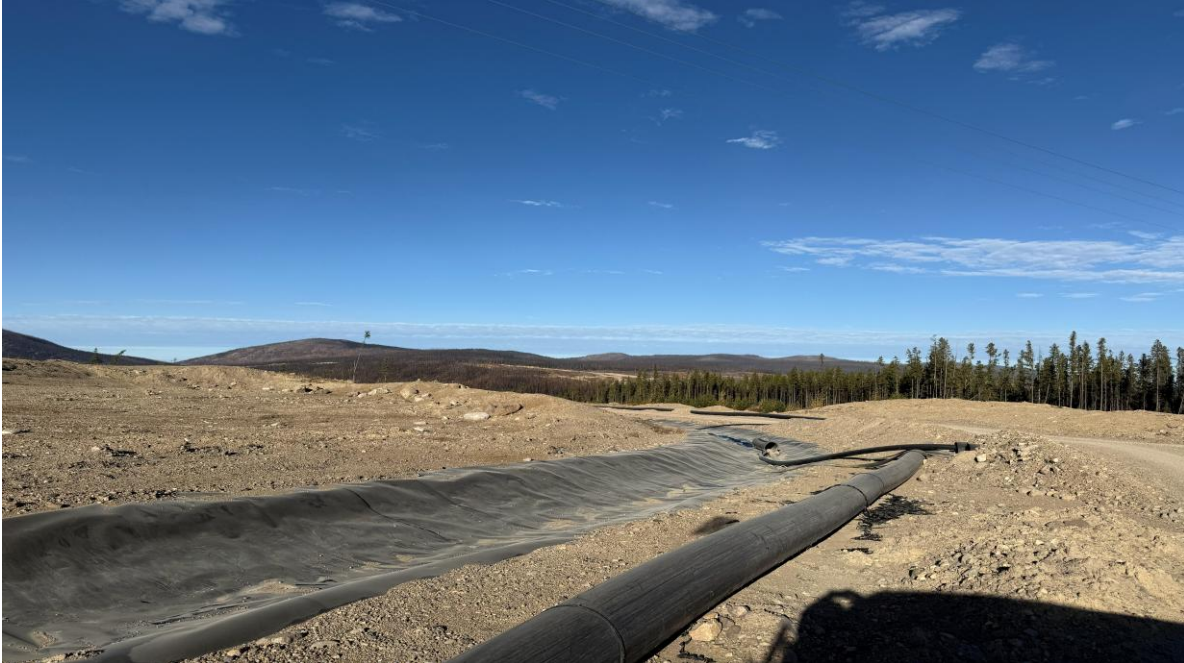
PHOTO 17 – SCC near its inlet and pipeline from Mine Area Creek sump and the WMP inlet, looking northwest (Photo taken on October 13, 2025)
