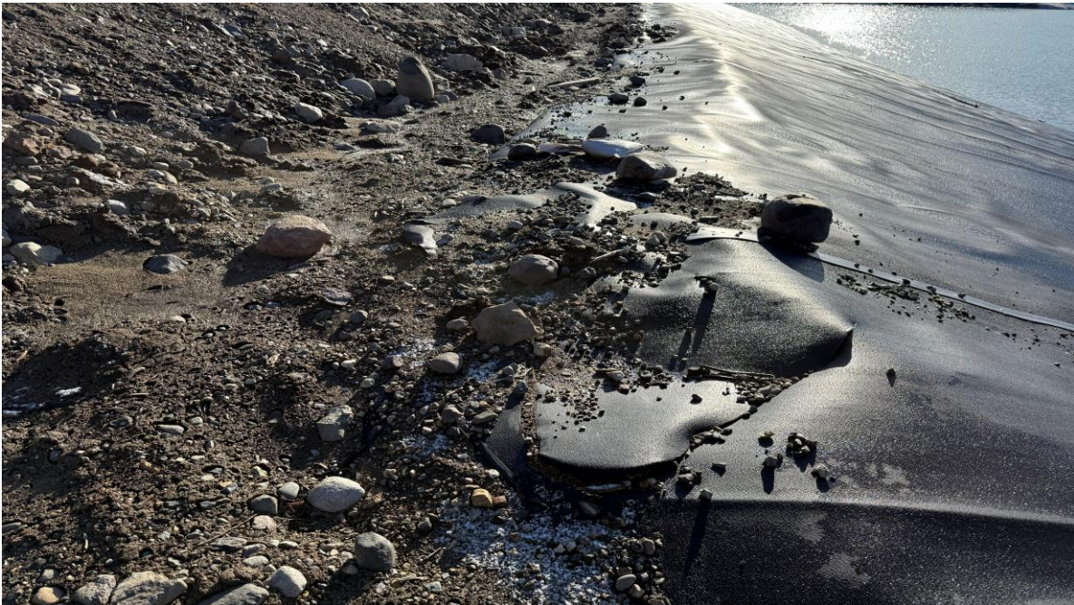
PHOTO 10 – IECD liner damage at the upstream crest, northwest corner (Photo taken on November 11, 2025)
