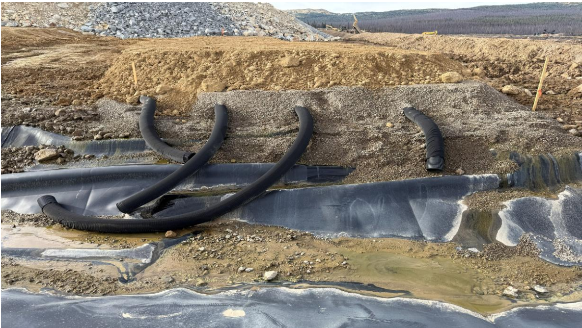
PHOTO 22 – LGO liner foundation drain outlet to MCC, looking south (Photo taken on September 15, 2025)
