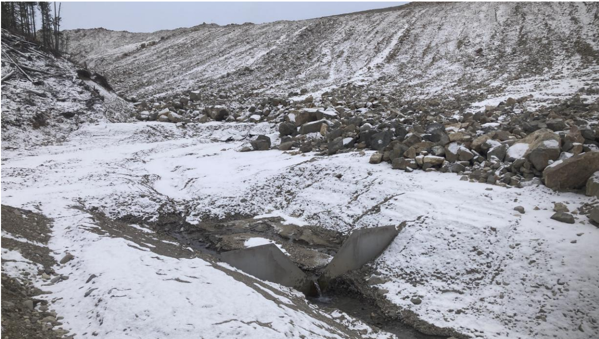
PHOTO 27 – East foundation drain and weir, looking east (Photo taken on November 28, 2025)
