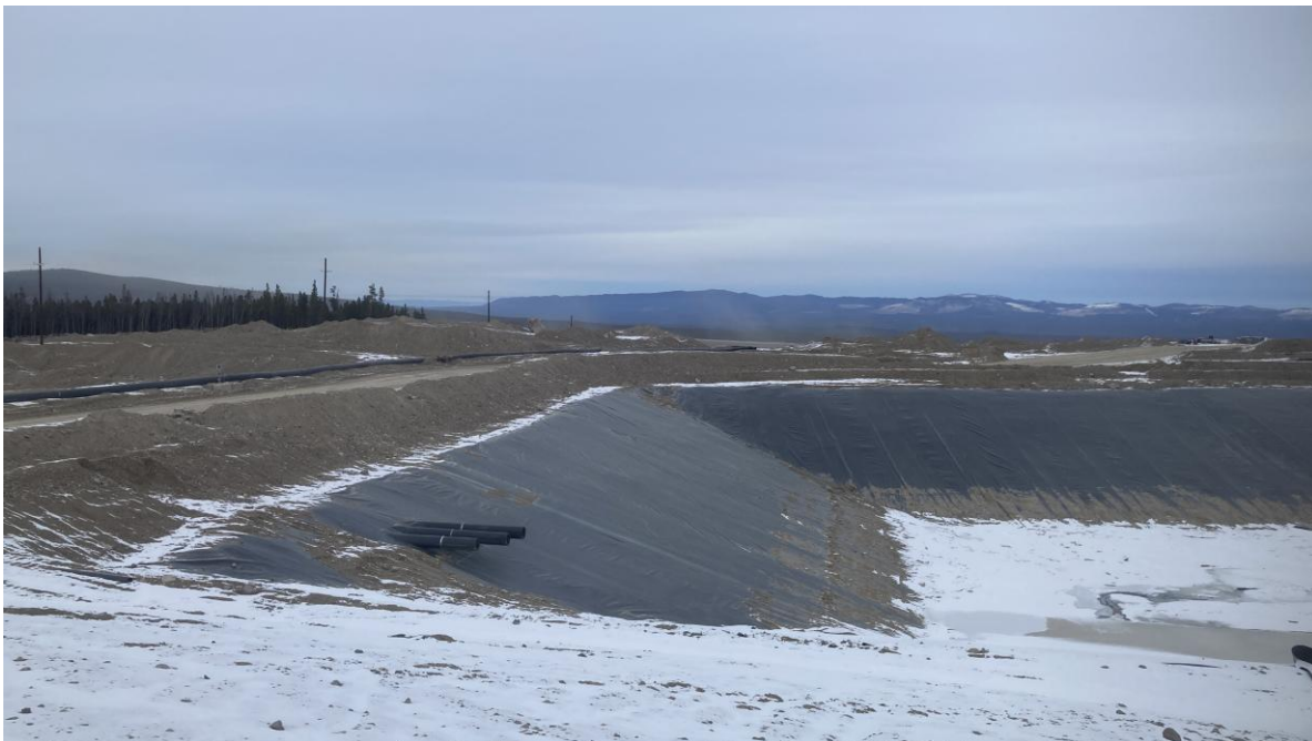
PHOTO 20 – West Berm upstream slope and West Berm Outlet pipes, looking north (Photo taken on November 28, 2025)
