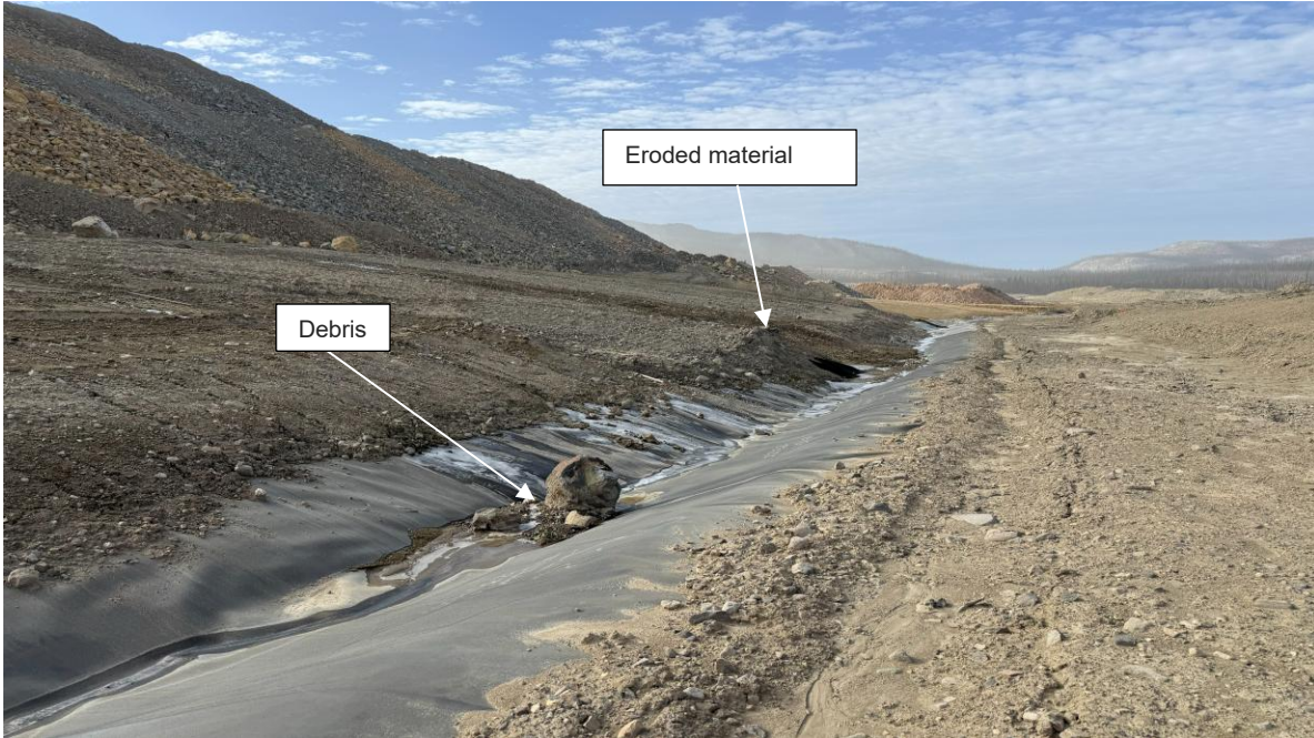
PHOTO 19 – MCC debris accumulation and minor sloughing into channel from the LGO foundation soil liner, looking west. Sloughed material was removed in November 2025 (Photo taken on October 13, 2025)
