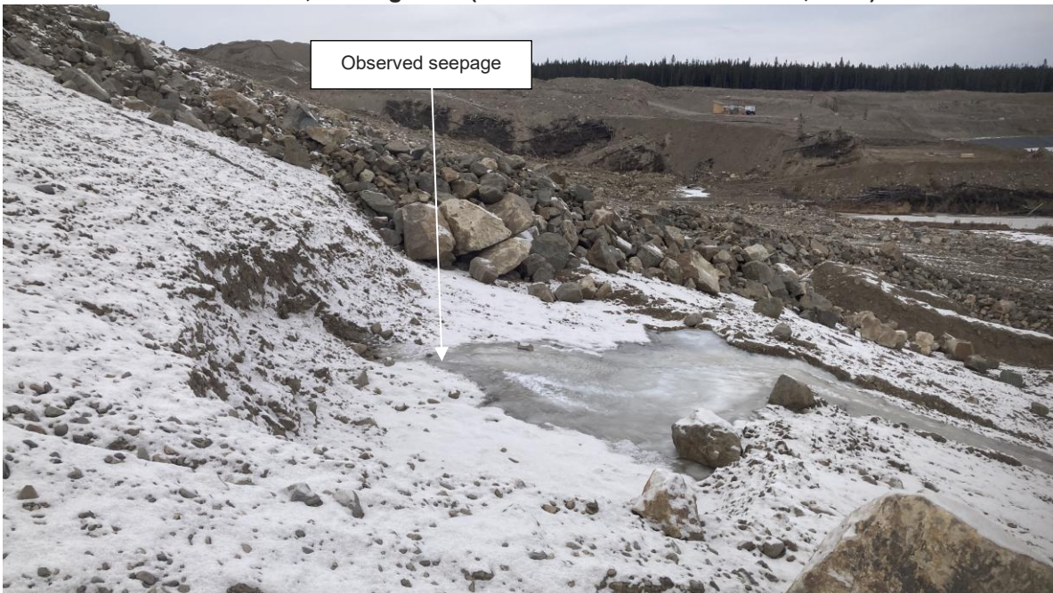
PHOTO 24 – Observed perched seepage discharging along the downstream slope of the buttress, looking northwest (Photo taken on November 28, 2025)
