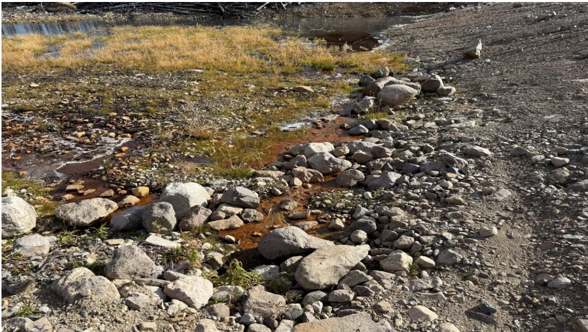
PHOTO 8 – Seepage observed at the downstream toe of Lake 16 Diversion Berm (Photo taken on October 13, 2025)
