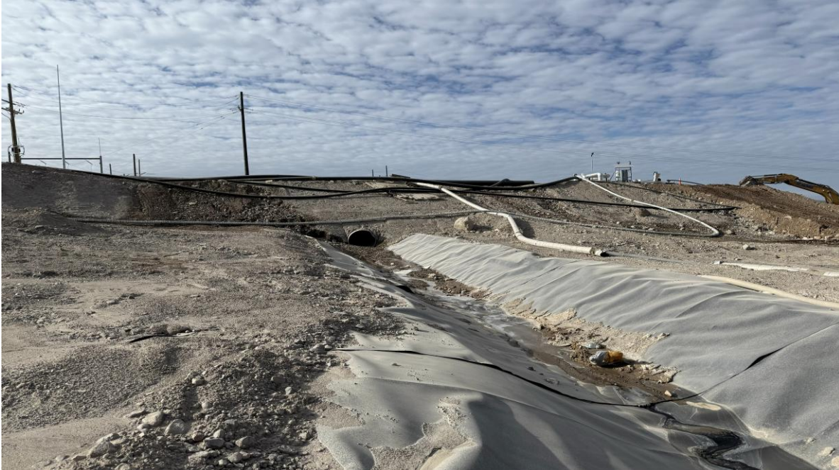
PHOTO 17 – North Collection Channel culvert (Photo taken on October 13, 2025)
