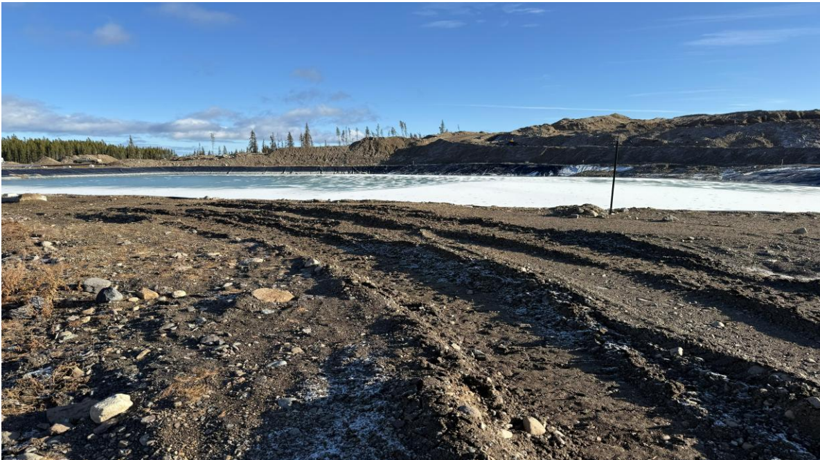
PHOTO 38 – TSF SCP west crest rutting, looking northwest (Photo taken on November 11, 2025)
