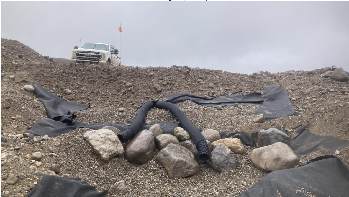
PHOTO 34 – West foundation drain outlet (Photo taken on May 17, 2025)
