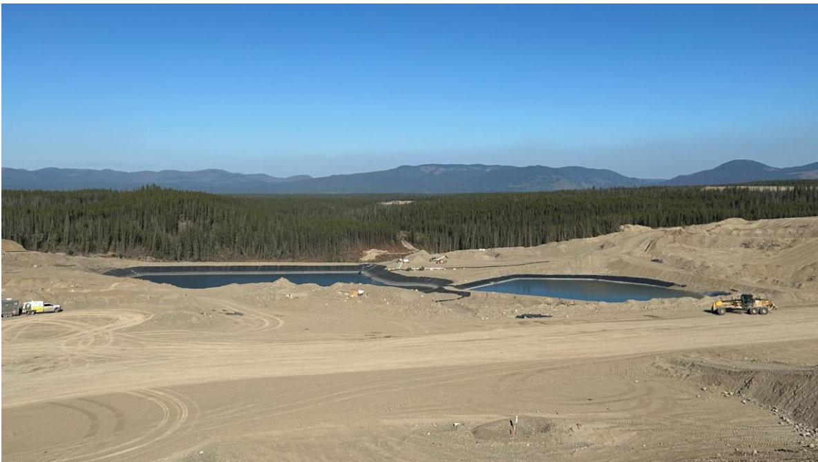
PHOTO 2 – IECD and TSF-SCP overview, looking northeast (Photo taken on September 18, 2025)
