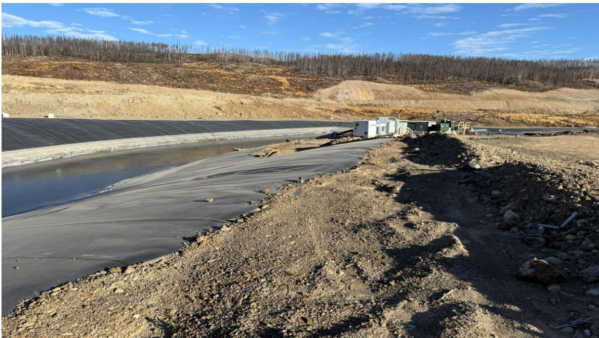
PHOTO 4 – CDS pump station, looking north (Photo taken on October 13, 2025)
