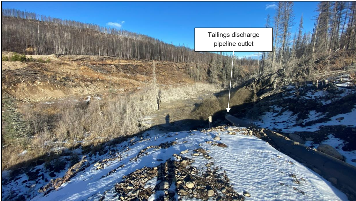
PHOTO 3 – Tailings discharge pipeline outlet, looking northeast (Photo taken on November 3, 2025)
