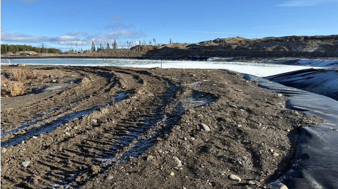
PHOTO 37 – TSF SCP west crest rutting, looking east (Photo taken on November 11, 2025)
