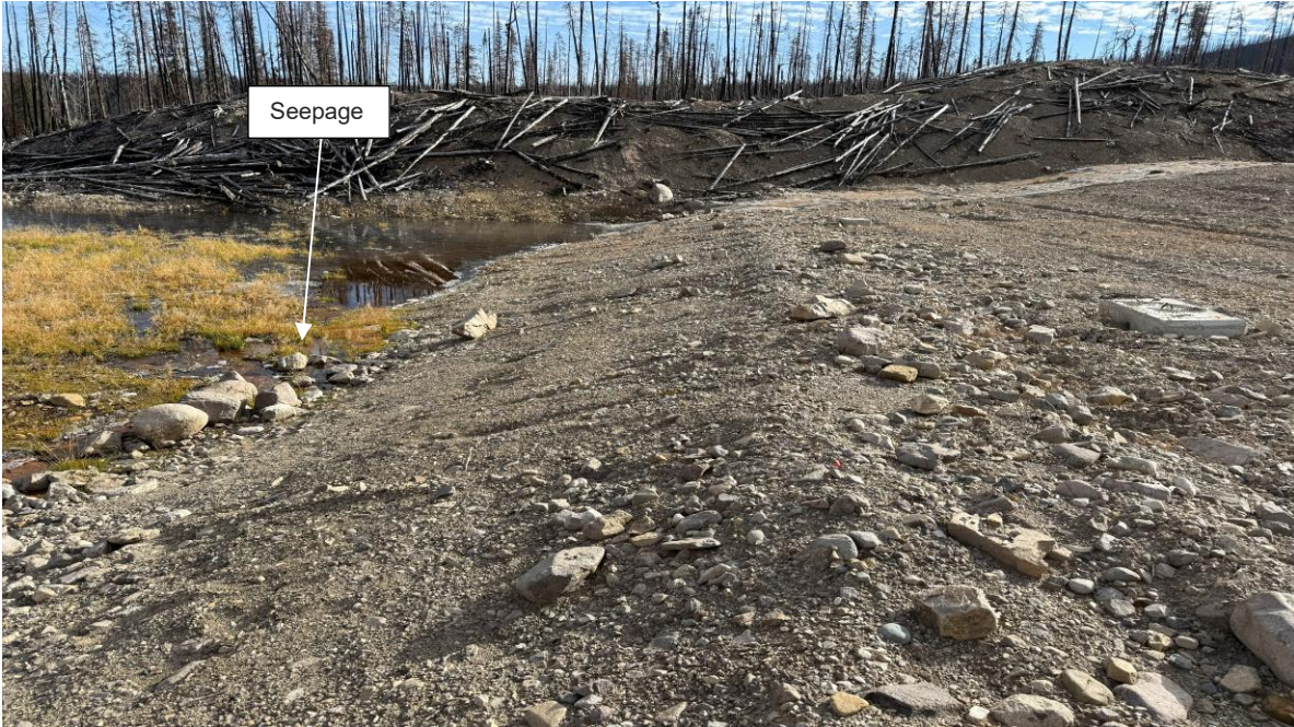
PHOTO 7 – Downstream slope and seepage, looking east (Photo taken on October 13, 2025)
