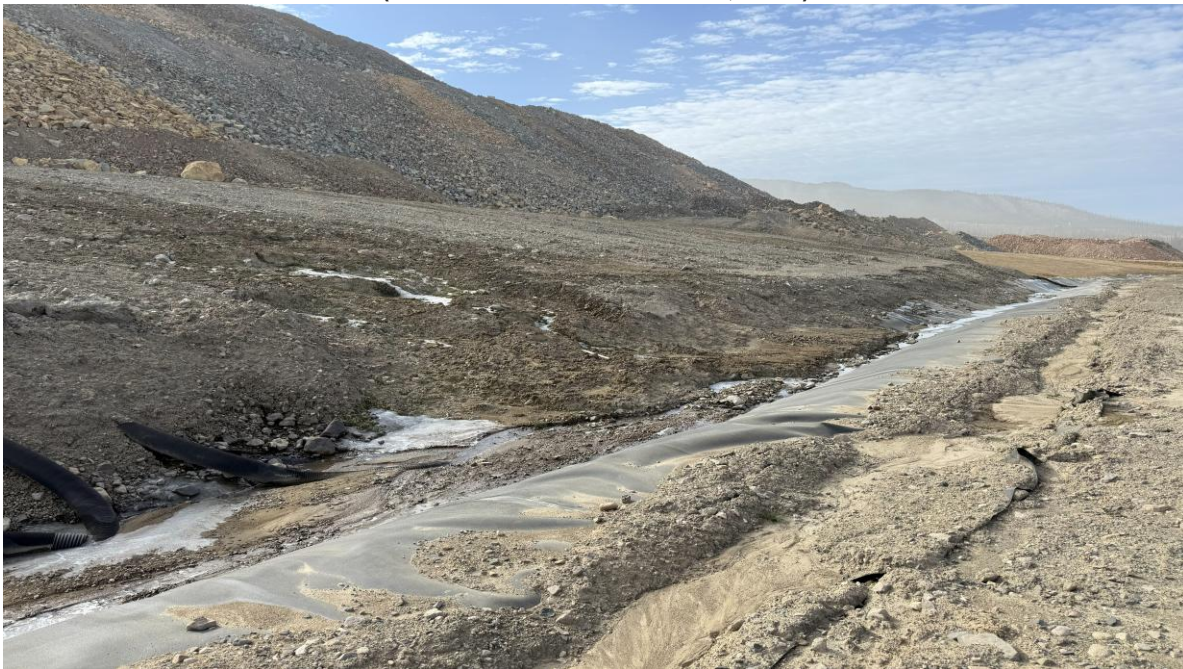
PHOTO 20 – Sloughing, sediment accumulation and anchor trench erosion along the MCC, looking west (Photo taken on October 13, 2025)
