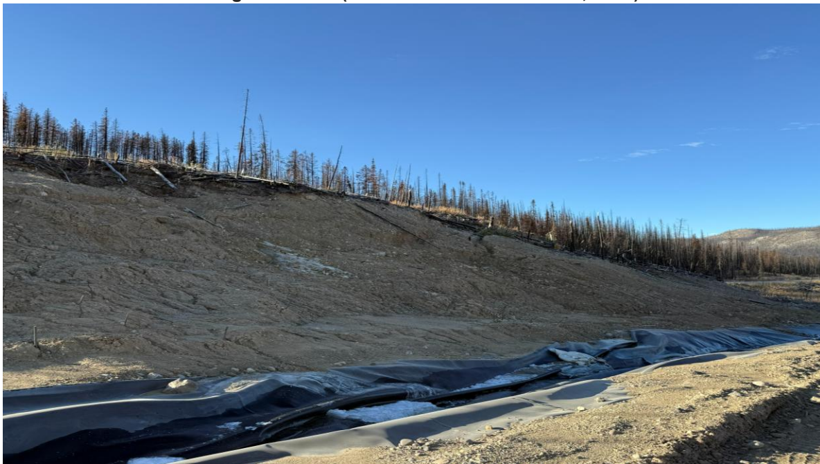
PHOTO 18 – SCC deformed liner, looking southwest (Photo taken on October 13, 2025)
