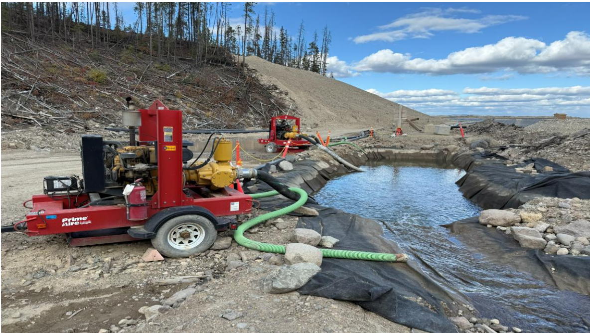
PHOTO 16 – Mine Area Creek sump and pumping system at the WMP inlet, looking north (Photo taken on October 11, 2025)
