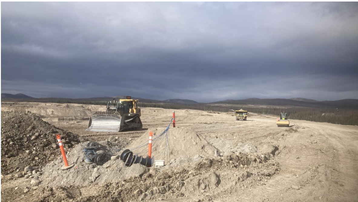
PHOTO 38 – MDC-S1W-PZ3 inclinometer and VWPs installed to 20 channel datalogger (Photo taken on Spetember 20, 2025)
