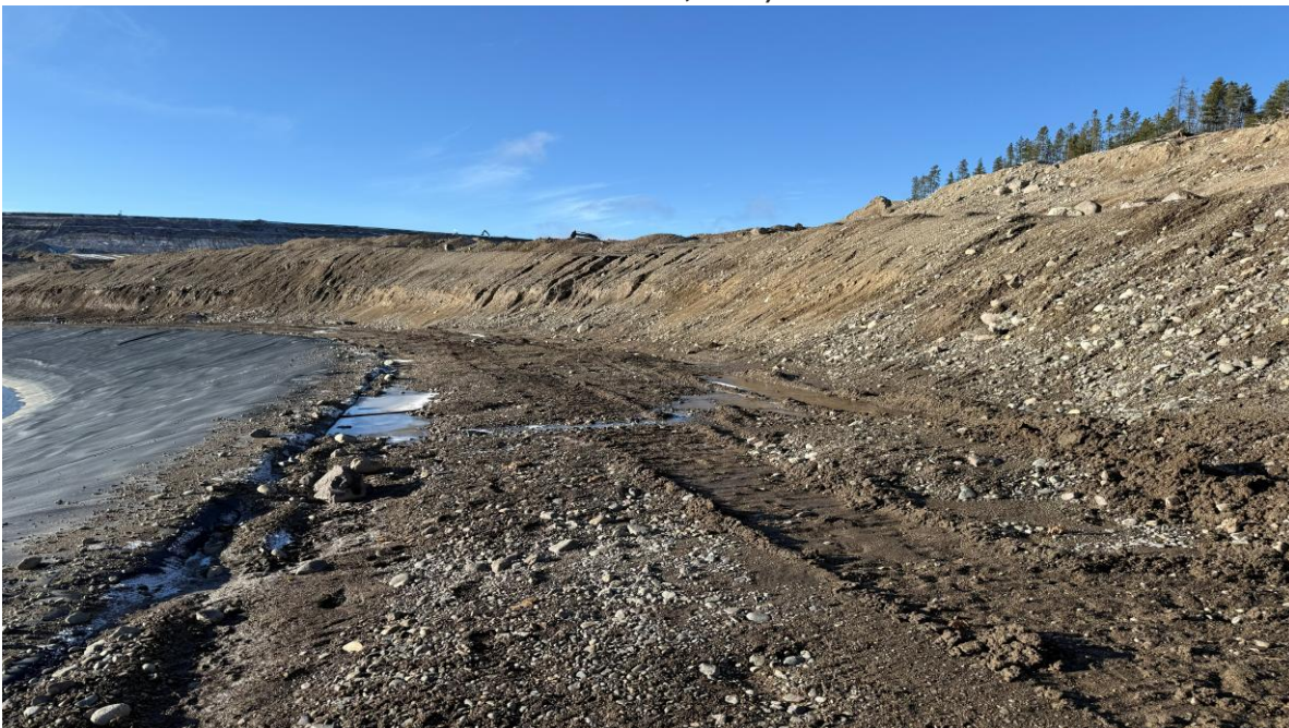
PHOTO 18 – IECD rutting and liner trench depressions along the northwest cut bench, looking southwest, (Photo taken on November 11, 2025)
