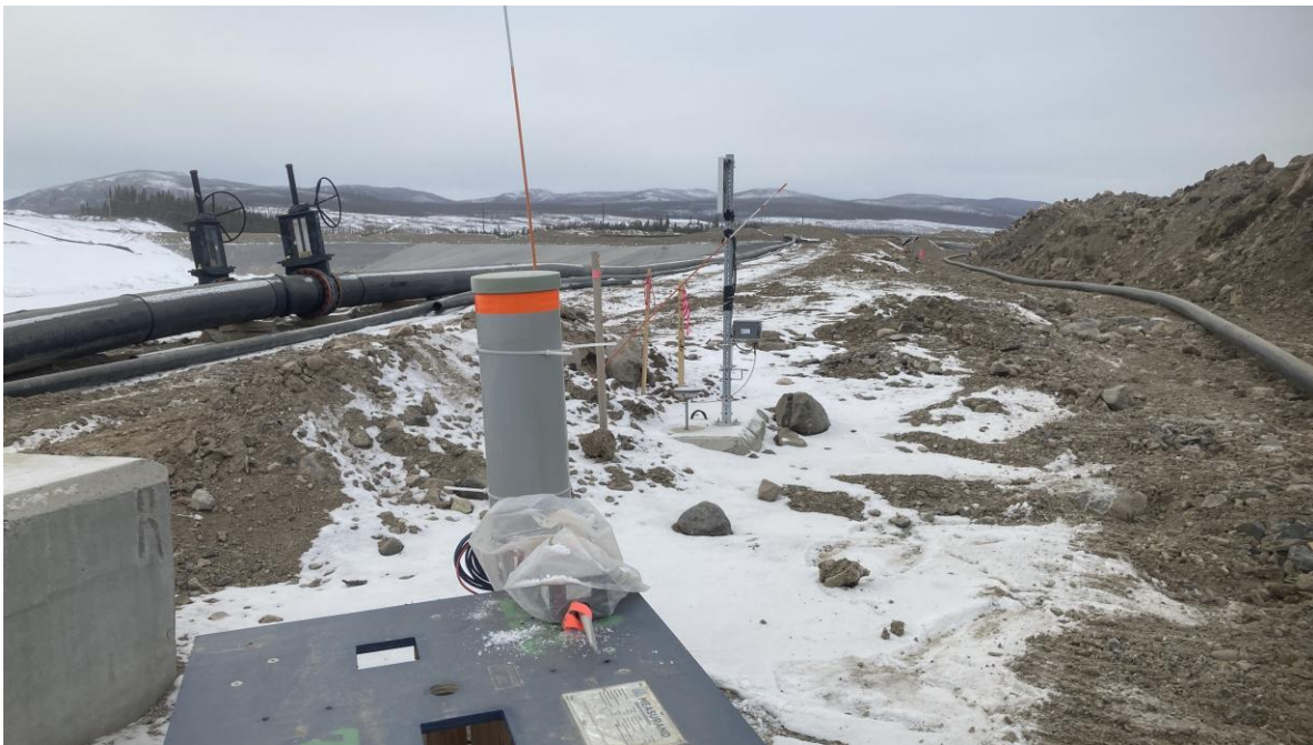
PHOTO 24 – North Berm pipeline and instrumentation (SAA and VWPs) (Photo taken on November 28, 2025)
