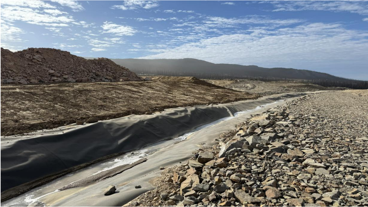
PHOTO 21 – MCC, looking southwest (Photo taken on October 13, 2025)
