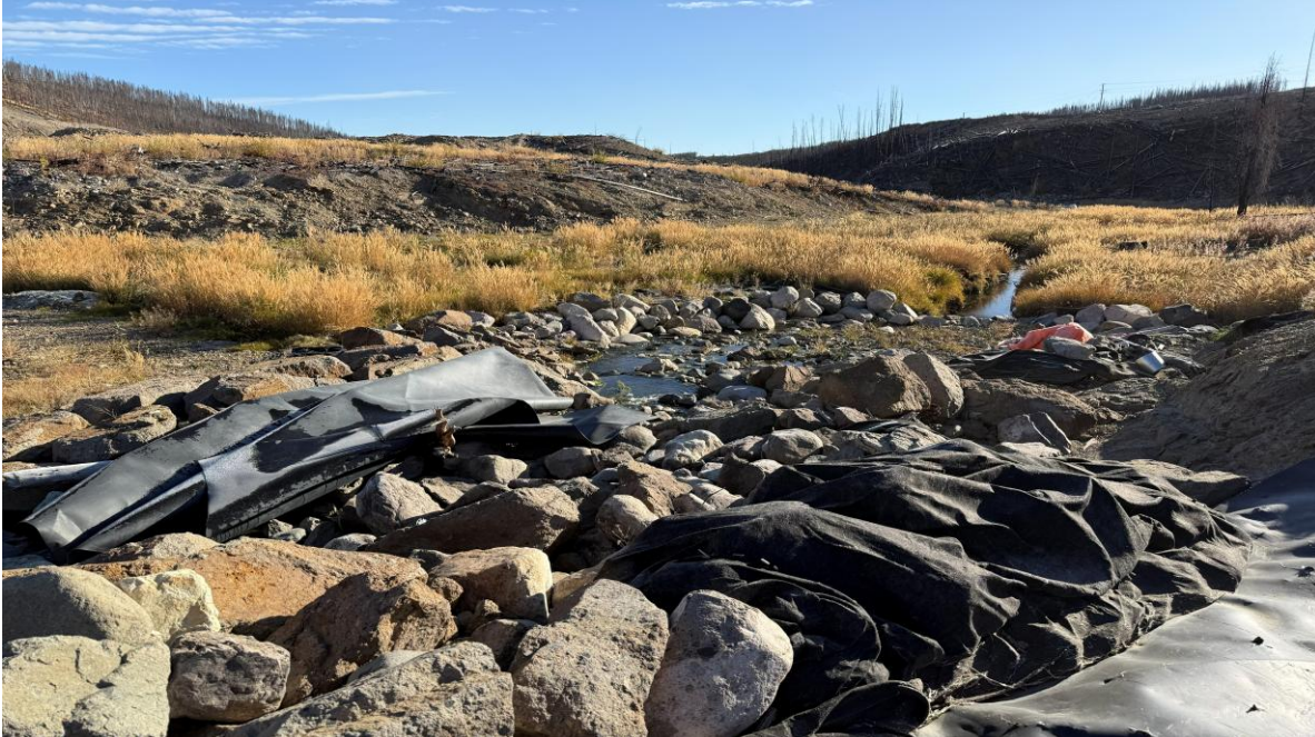
PHOTO 13 – CWTP spillway stilling basin and deformed HDPE liner, looking northeast (Photo taken on October 13, 2025)
