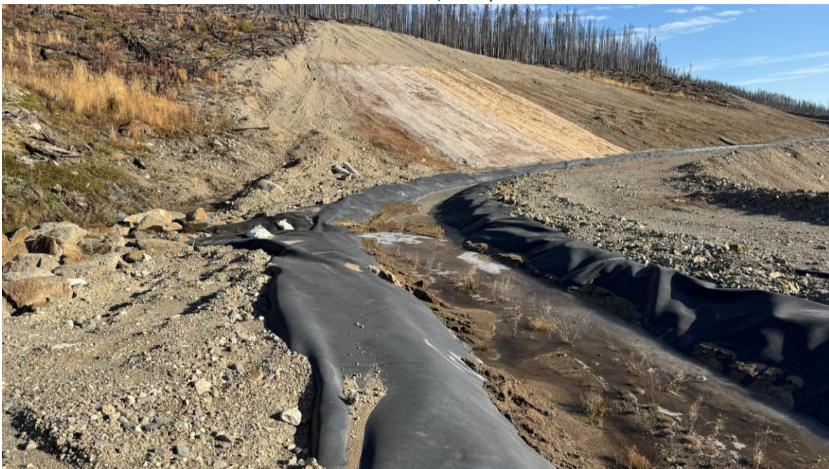
PHOTO 20 – Sediment accumulation in the NCC, looking north (Photo taken on October 13, 2025)
