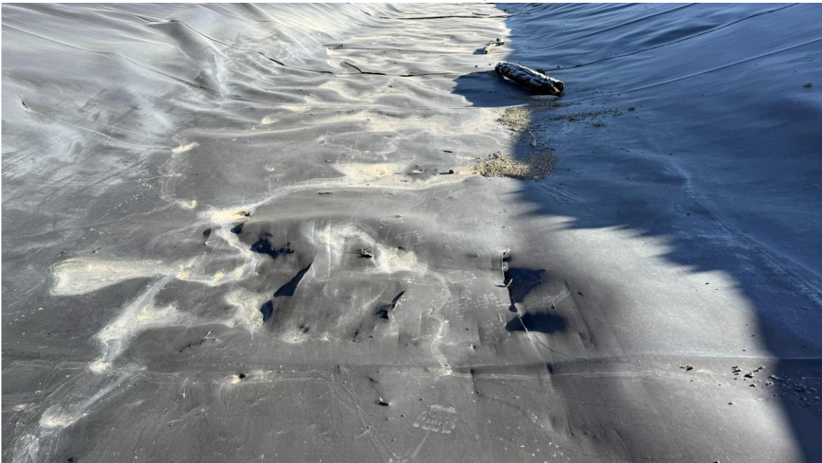
PHOTO 12 – CWTP spillway HDPE liner damage (Photo taken on October 13, 2025)
