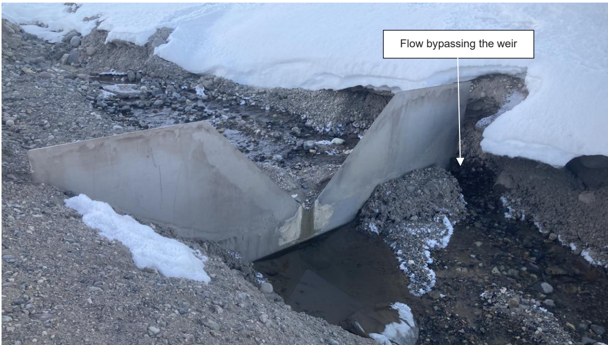
PHOTO 33 – Seepage flow bypassing the east foundation drain weir (Photo taken on January 24, 2026)
