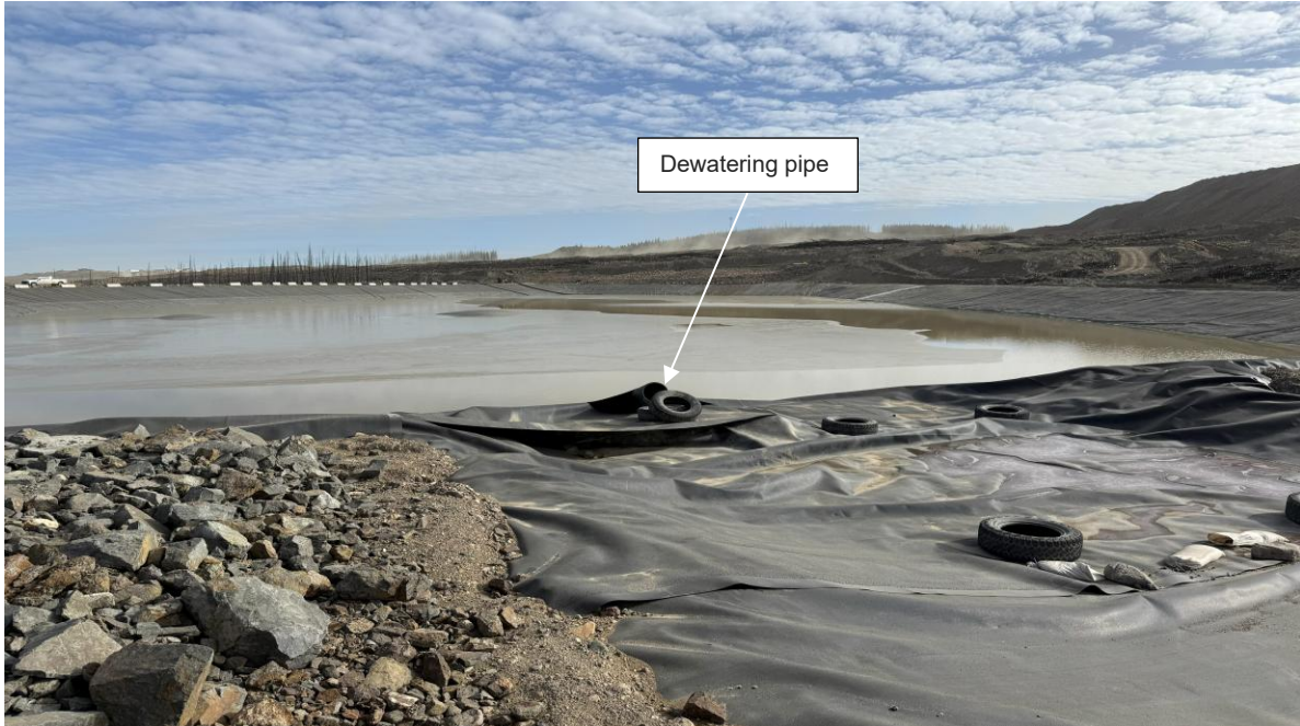
PHOTO 13 – LGO CP spillway inlet and HDPE liner; under liner dewatering pipe, looking west (Photo taken on October 13, 2025)
