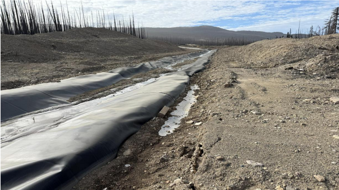
PHOTO 17 – WCC sediment accumulation and anchor trench settlement, looking southwest (Photo taken on October 13, 2025)
