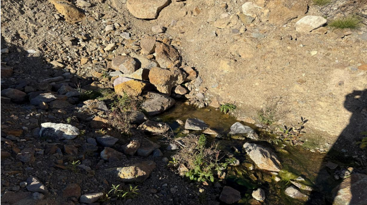
PHOTO 9 – CWTP foundation drain outlet (Photo taken on October 13, 2025)
