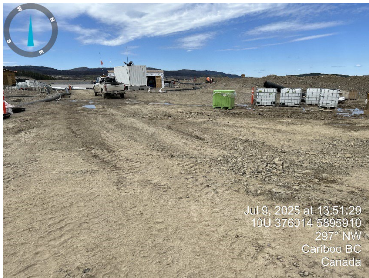
Photo 6: Spill Clean Up
