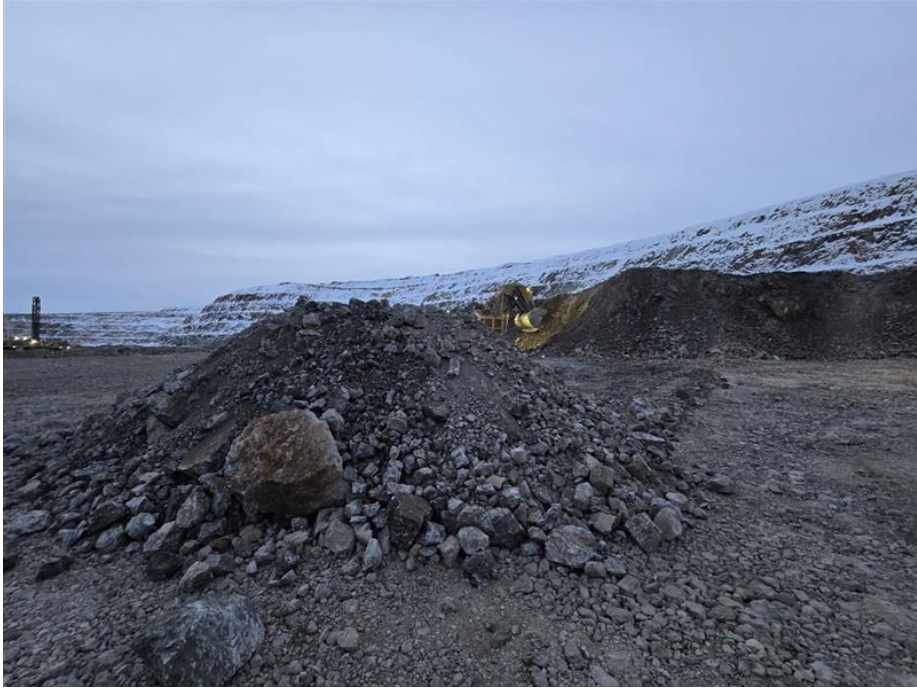
Photo 5: Contaminated material pile prior to removal
