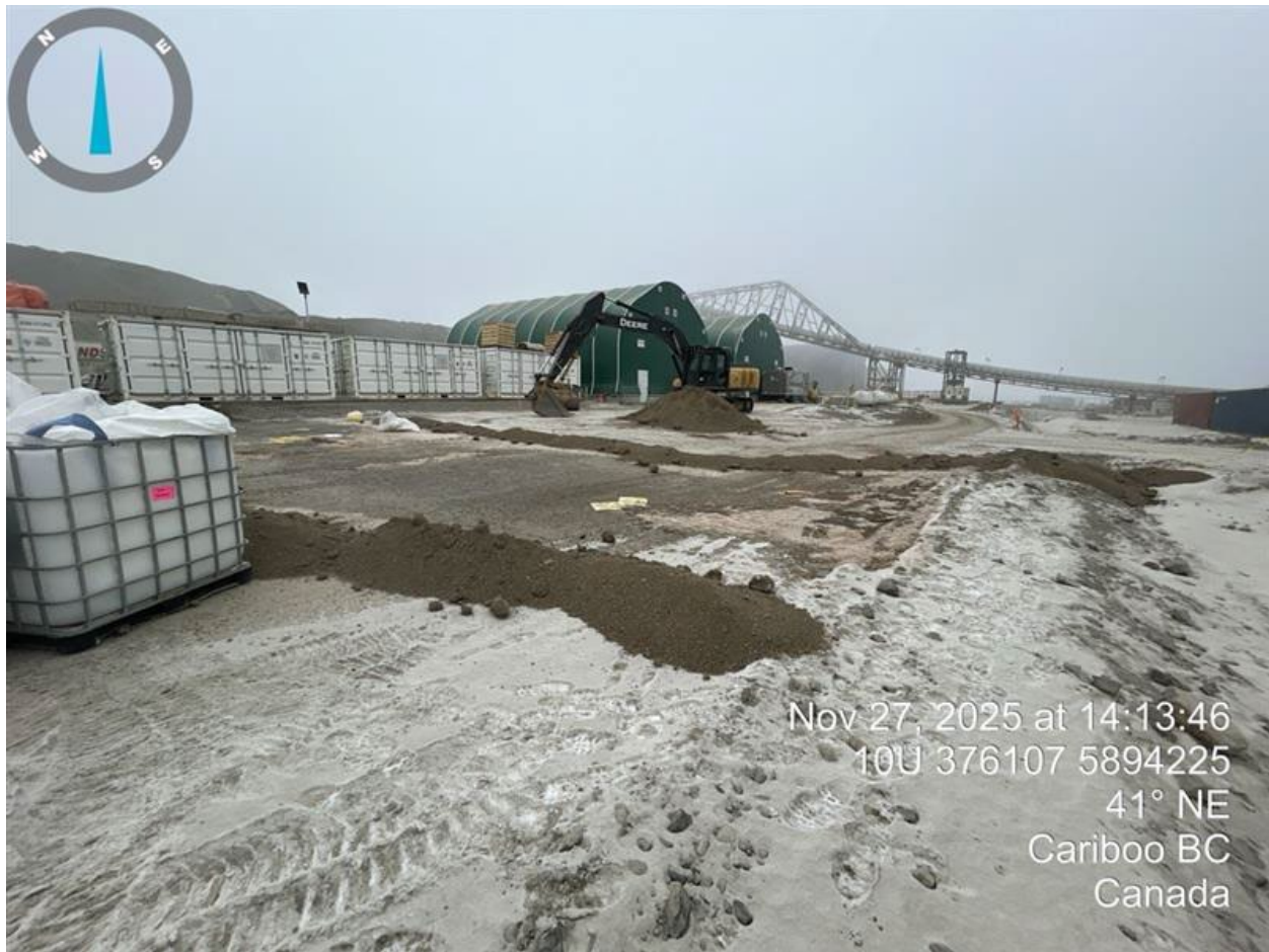
Image 3: Temporary berm constructed to provide tertiary containment for the spill.
