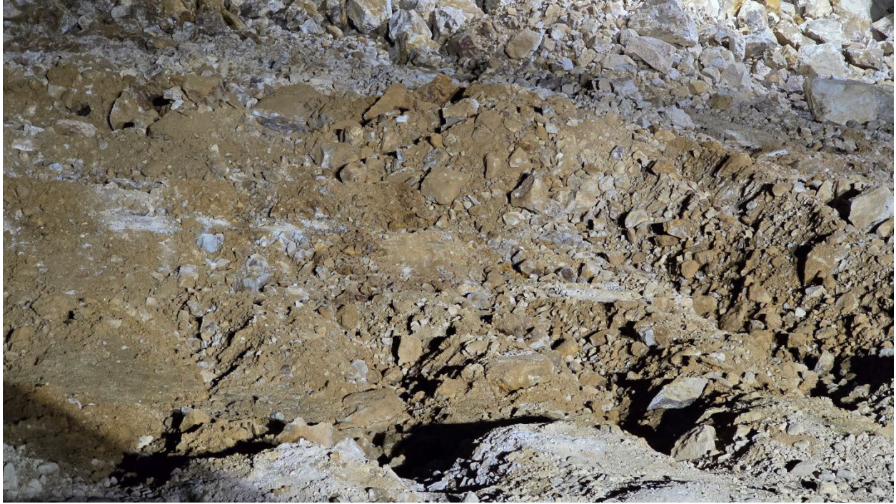
Photo Three: Spill Clean Up Closeup
