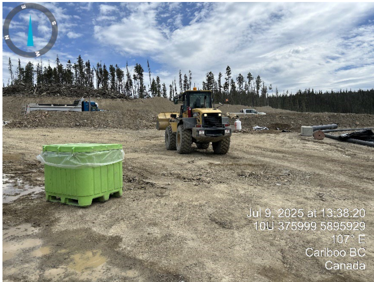
Photo 4: Spill Cleanup Ongoing
