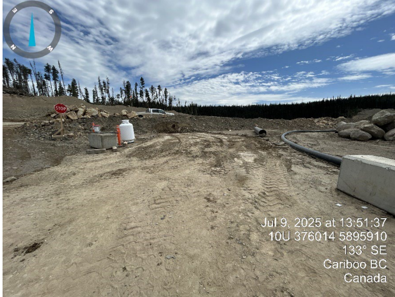
Photo 7: Spill Clean Up
